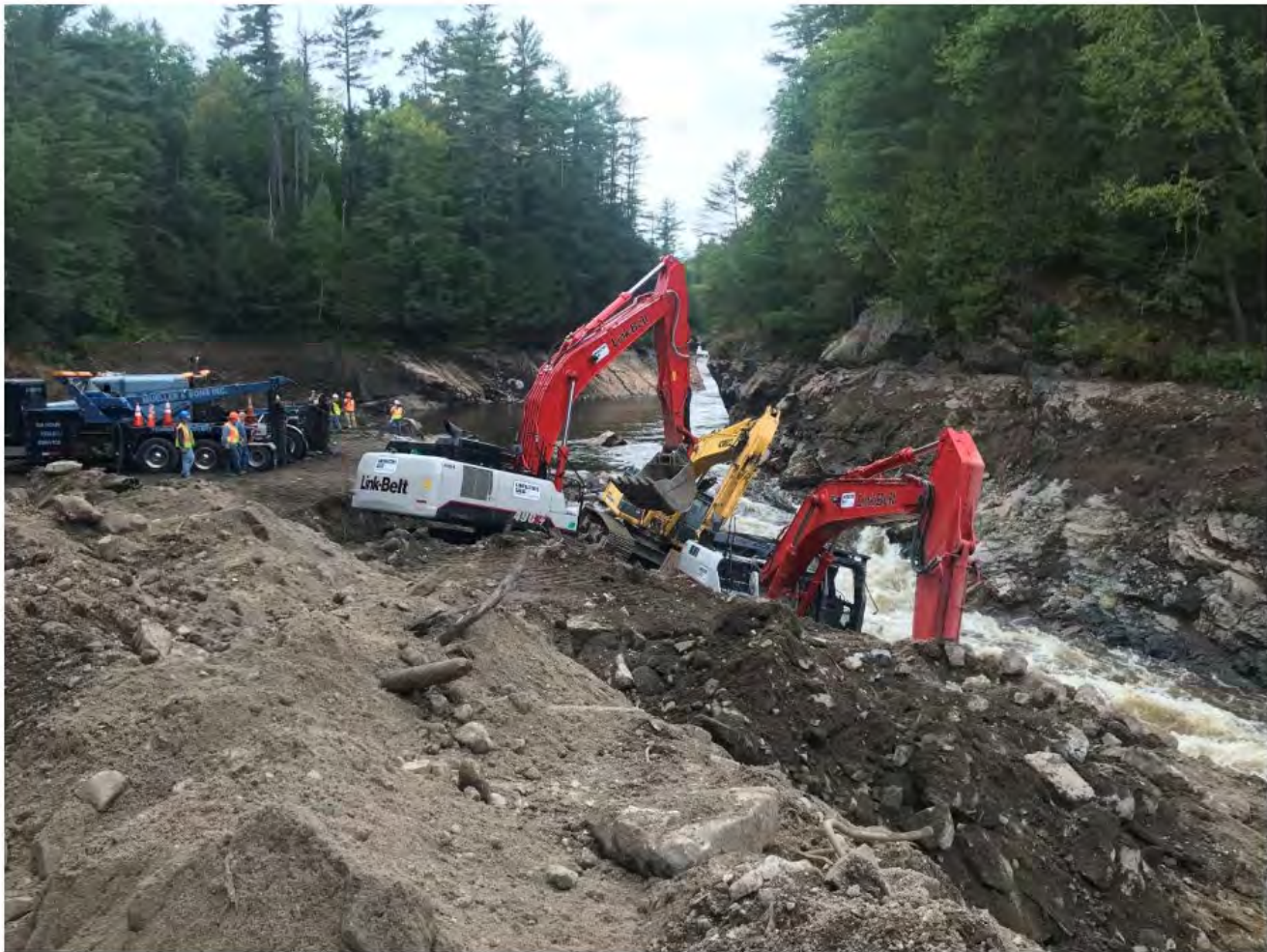
Two excavators at the edge of the pilot channel that were toppled in flood waters and uprighted.
