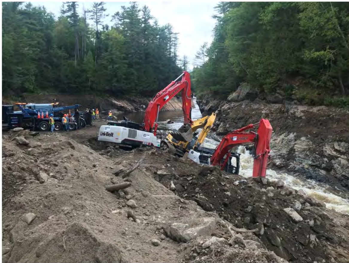
Two excavators at the edge of the pilot channel that were toppled in flood waters and uprighted.
